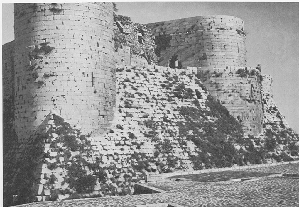
LIII. Krak des Chevaliers: a. view from the west b. the southern talus
